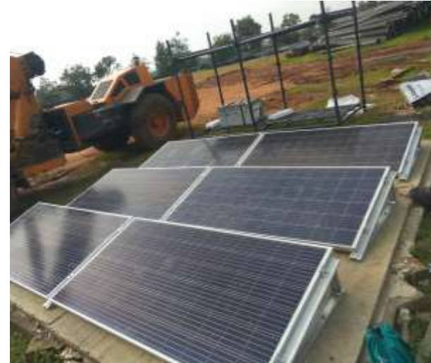
Solar Off-Grid system
