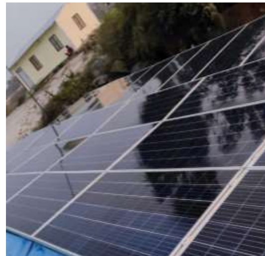
Solar On-Grid system
